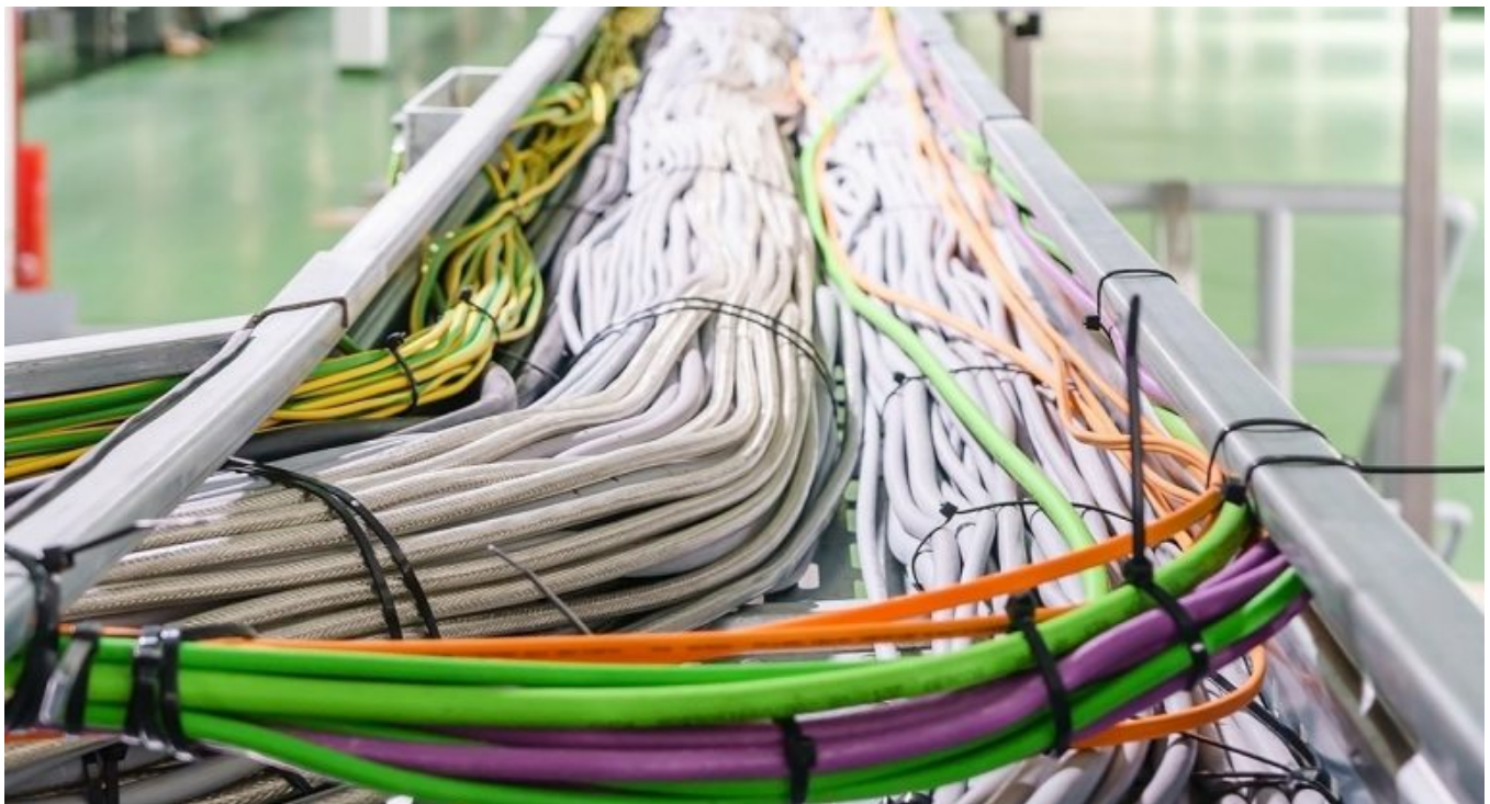
Traditional Category Cable Network
